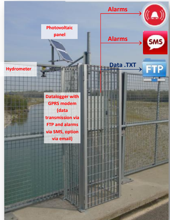
Surface water monitoring and alarm station
