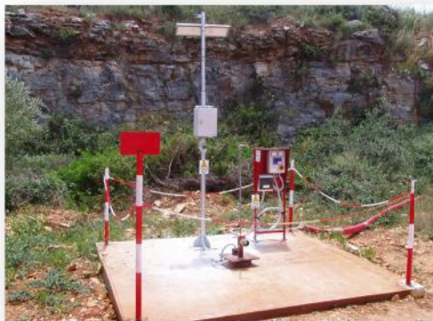
Underground water monitoring station in a landfill
