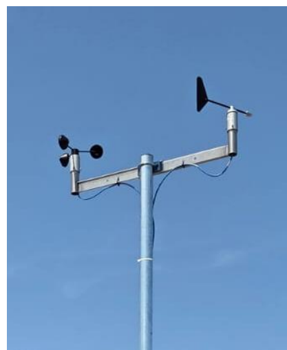
Typical installation on weather and environmental stations
