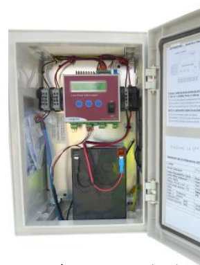
Datalogger mounting in the IP65 container
