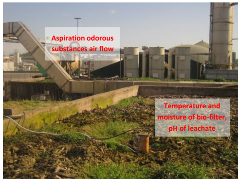
Temperature-moisture, pH and air aspiration monitoring in a bio-gas plant
