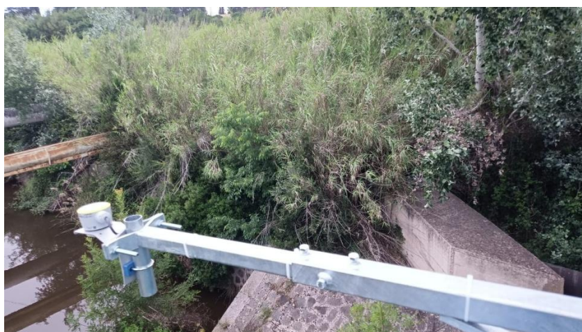
Picture 1 – Installation example of a hydrometric station with radar sensor
