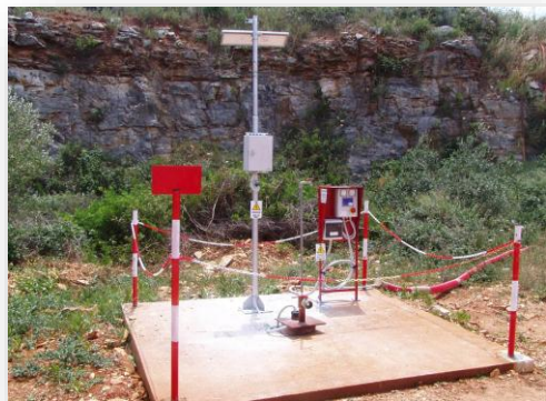
Underground water monitoring station in a landfill
