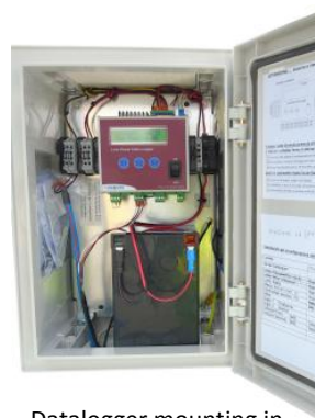
Datalogger mounting in the IP65 container
